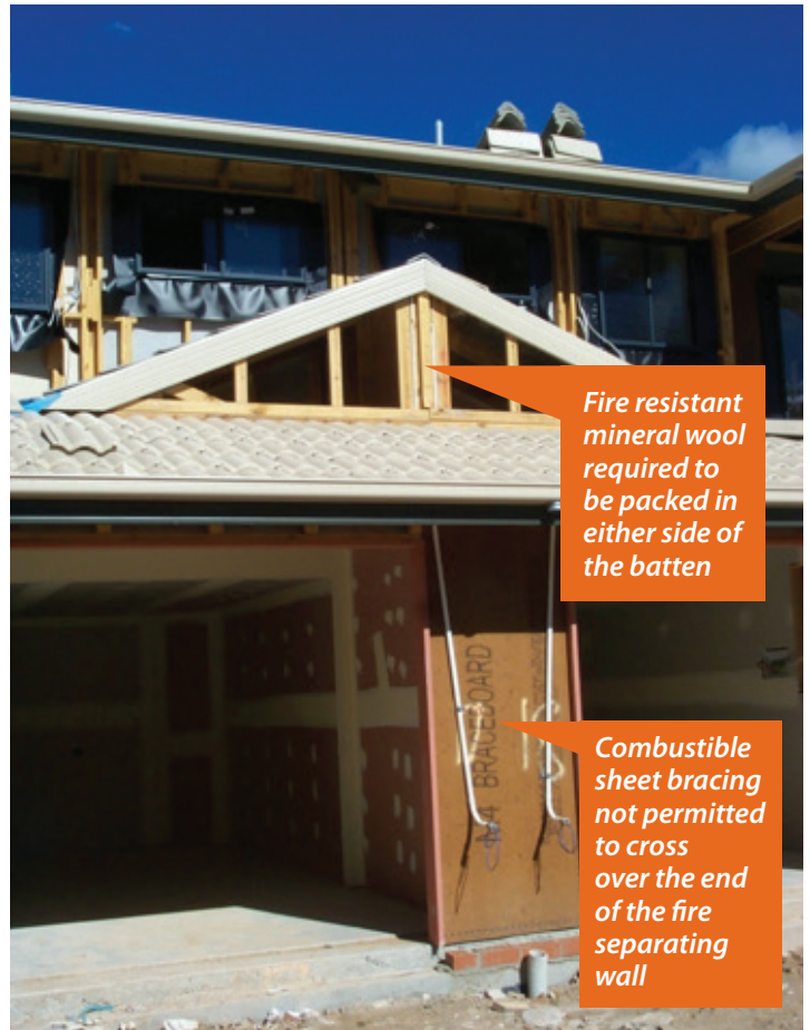
Photograph 4. Separating wall extends out through Dutch Gable. To comply, the vertical batten on the end of the wall will require fire resistant mineral wool to be packed into the end cavity either side of the batten.
