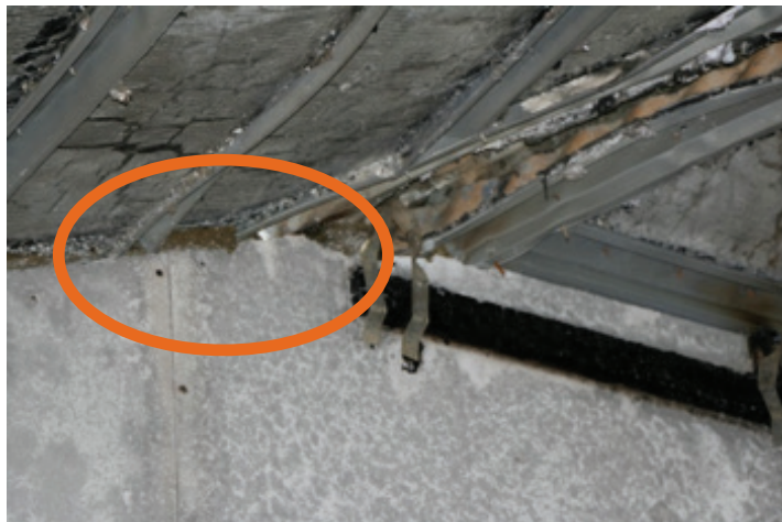
Photograph 1. Fire damaged unit. Note: gaps between battens filled with mineral wool to prevent fire spread across separating wall.
