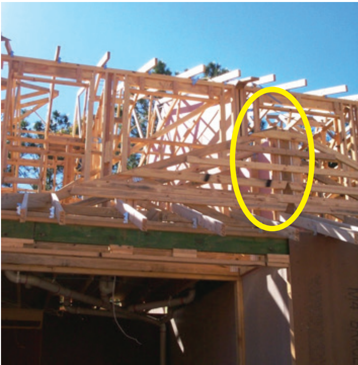
Photograph 3. Separating wall extends out through Dutch Gable, however the framing members that cross the end of the Dutch Gable will not comply with the fire separating wall requirements.
