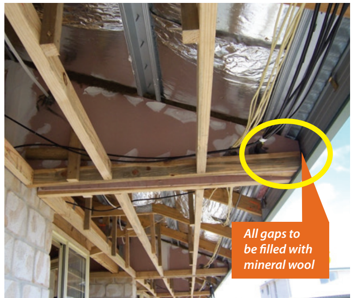
Photograph 5. All spaces are required to be filled with fire resistant mineral wool or other fire rated material including under all top hat battens, behind fascias and to the end of the separating wall.
