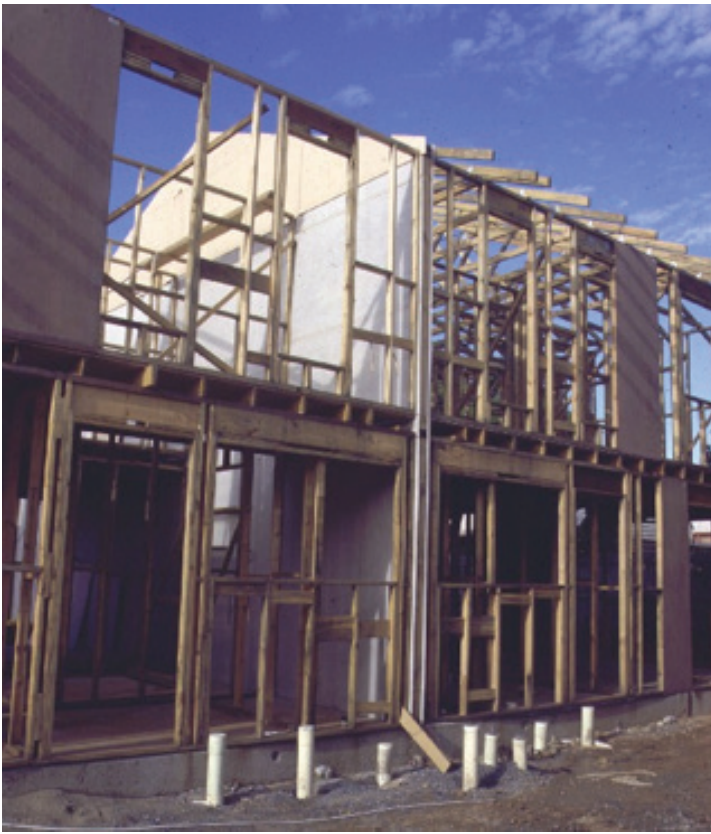
Photograph 2. Fire rated plasterboard extends beyond outside of external wall frame and into cavity. End of separating wall to be fitted with fire resistant mineral wool and DPC.
